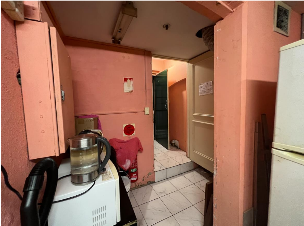
Figure 7: Basement level of the subject site showing staff entry and egress from Kent Street and stair access to the ground floor
